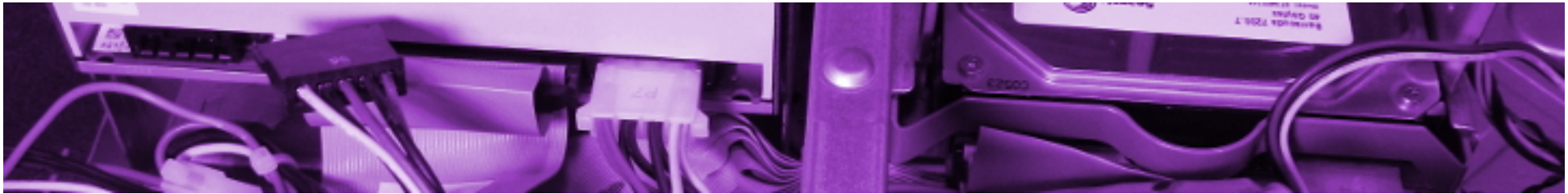
The guts of an IBM desktop PC circa 1995: cables carrying electrical current and those carrying data are both visible
